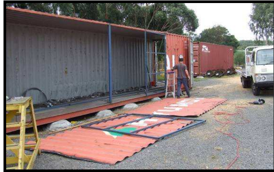
Frank Schroeders modifies one of the storage containers to enable it to be used to store motors. Photo – Anthony Smith.
