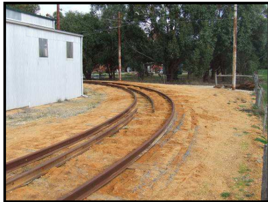
The rolled rail is prepared for welding and bolting to form up the north-west curve. Photo – Anthony Smith.
